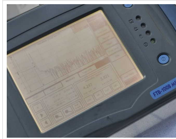
Singlemode and multimode optical testing
